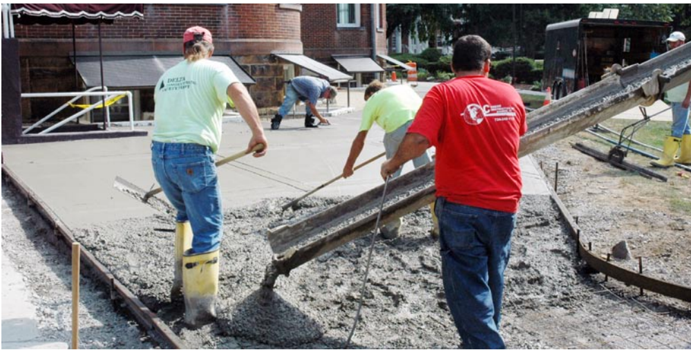
LAYING NEW TRACKS: It was smooth, cold and hard during the recent warm weather as cement masons poured and formed new sidewalks around Old Main. Crews took more than a week to tear out old sidewalk segments and curbing, before putting down new walkways. Work is now complete, and the sidewalks are open.
